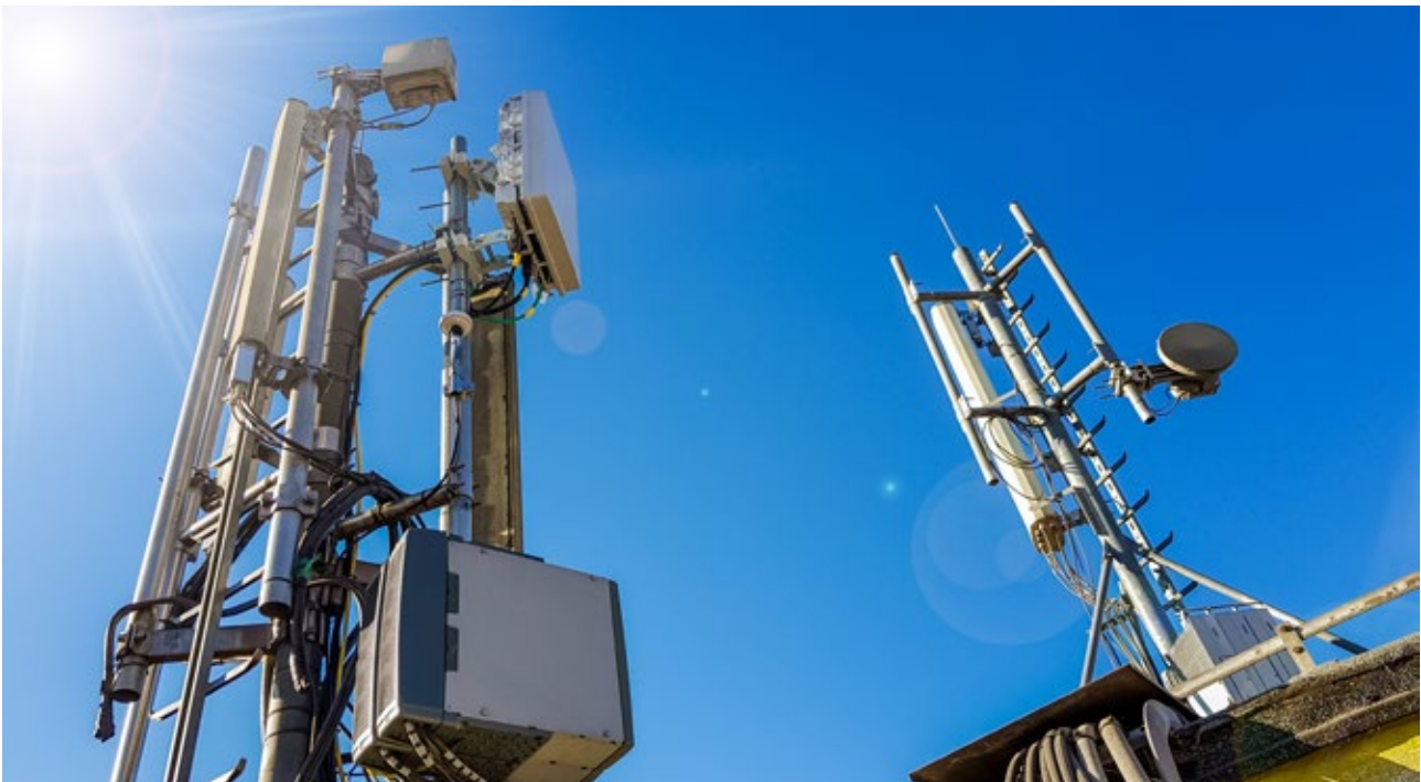
5G towers of a mobile telephony observatory in Paris.
